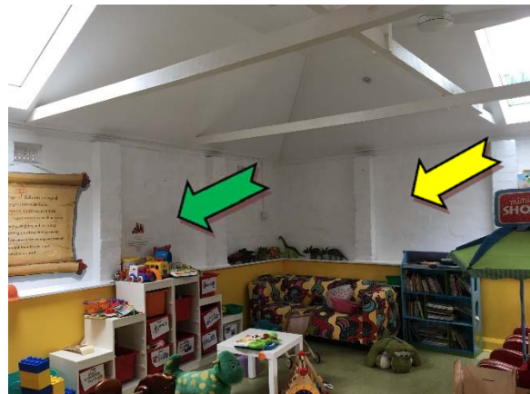
Photo 4. Interior, throughout, walls – suspected non asbestos-containing material and suspected lead-containing white upper paint system.
