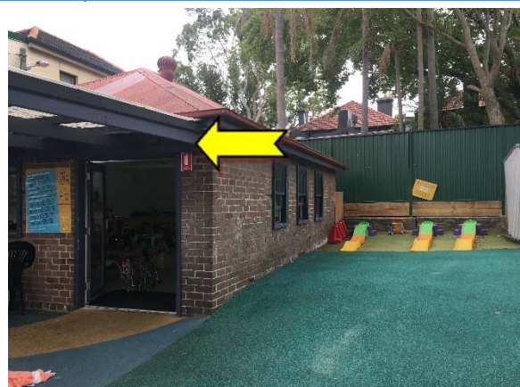
Photo 6. Exterior, throughout, timber supports – suspected lead-containing grey upper coloured paint systems.
