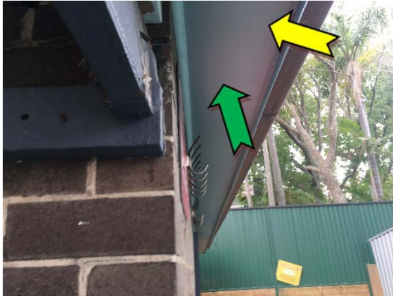
Photo 1. Exterior, throughout, eaves – non asbestos-containing fibre cement sheeting and suspected lead-containing white upper paint system.
